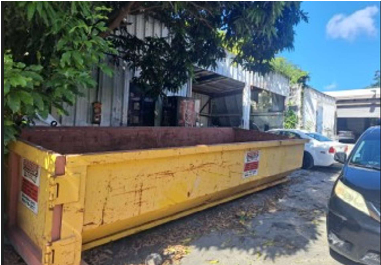
Site photo- Current condition of damaged building on property
