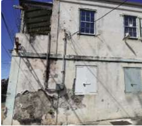
Before — Deteriorated side wall
