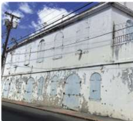
Before — Crumbling façade
