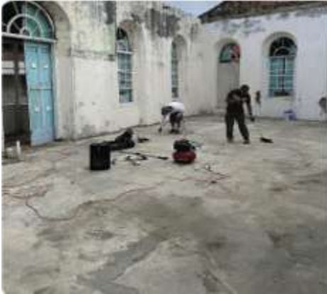
Before — Deteriorated exterior
