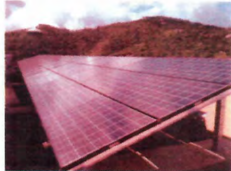
Photovoltaic Array Grandview Apartments, St. Thomas
