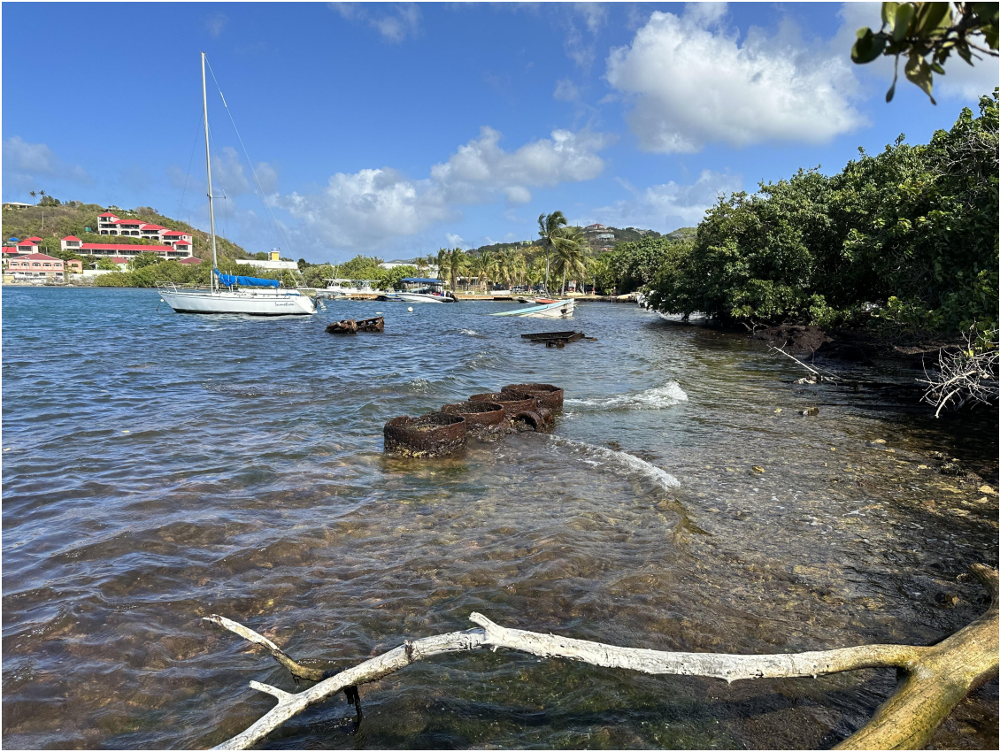
VIEW OF DAMAGED MARINA STRUCTURE LOOKING SOUTH
