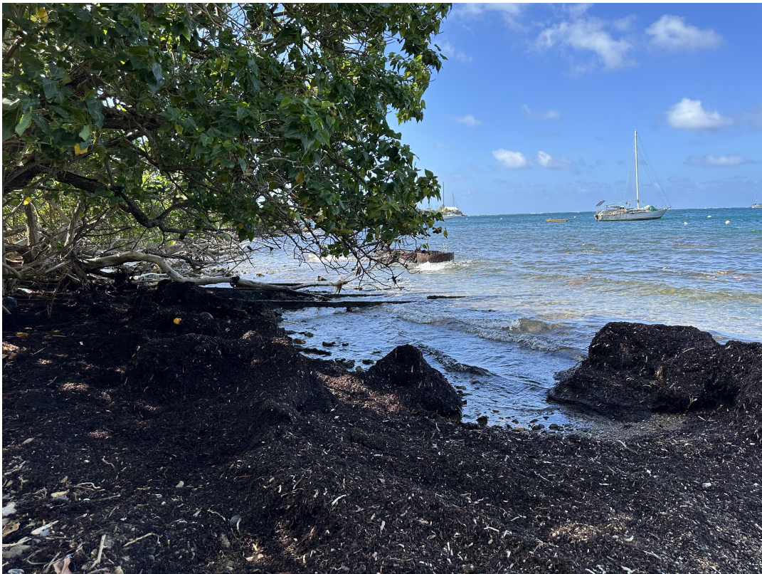
VIEW OF DAMAGED MARINA STRUCTURE LOOKING NORTH EAST
