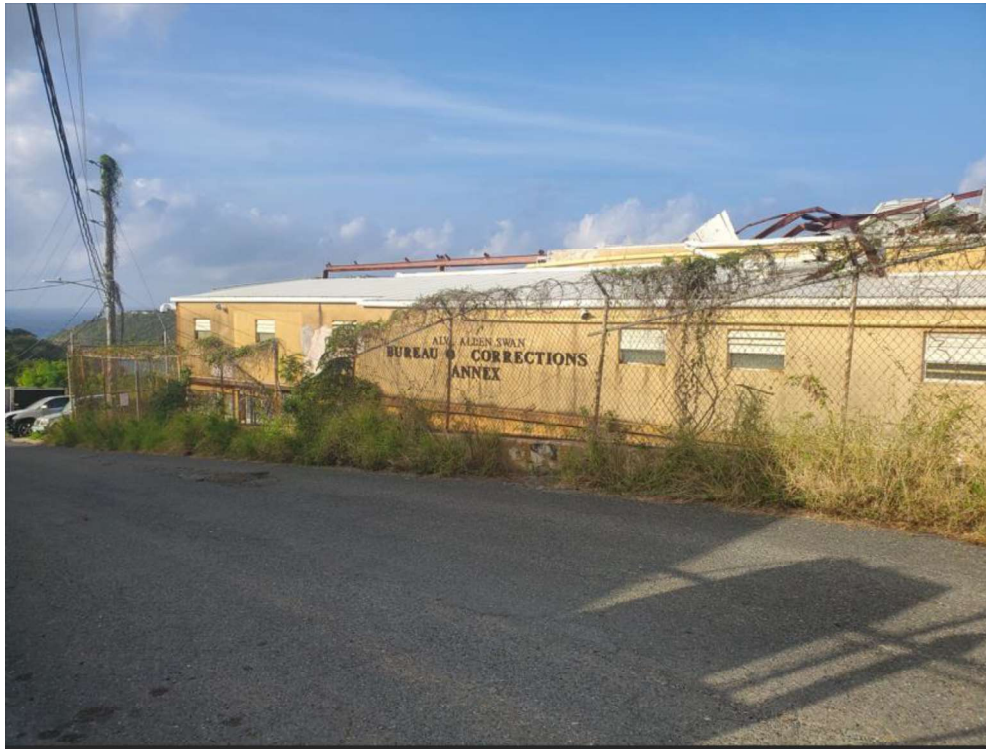
Photo of current site condition- hurricane damaged correctional institution
