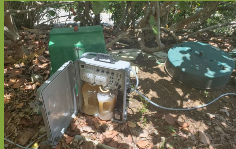
On-site Wastewater Disposal System
