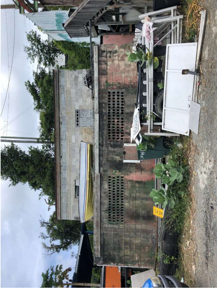
Figure 9: Hurricane Damaged Maintenance Building
