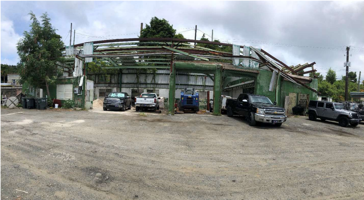
Figure 2: Hurricane Damaged Maintenance Building
