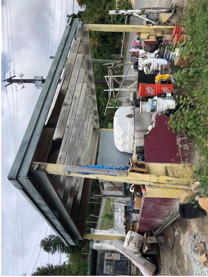
Figure 10: Hurricane Damaged Maintenance Building
