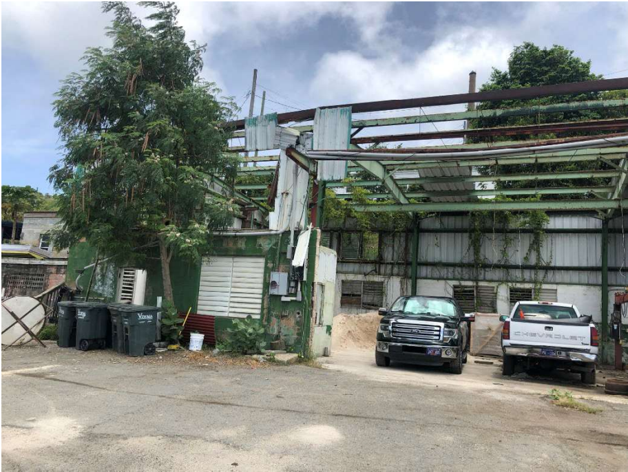
Figure 5: Hurricane Damaged Maintenance Building
