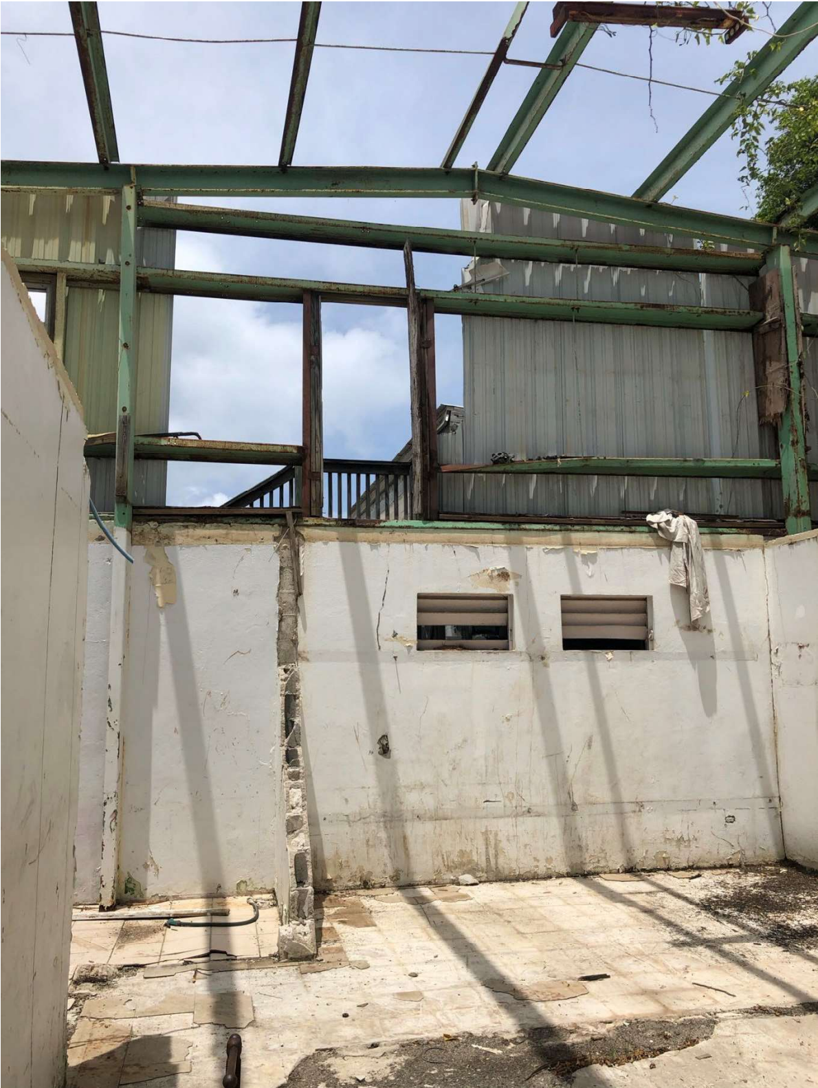
Figure 7: Hurricane Damaged Maintenance Building
