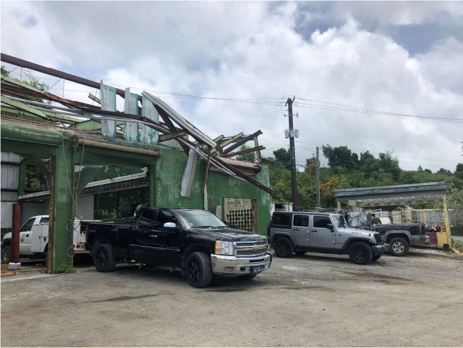
Figure 4: Hurricane Damaged Maintenance Building
