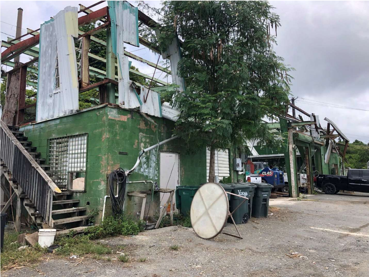
Figure 8: Hurricane Damaged Maintenance Building
