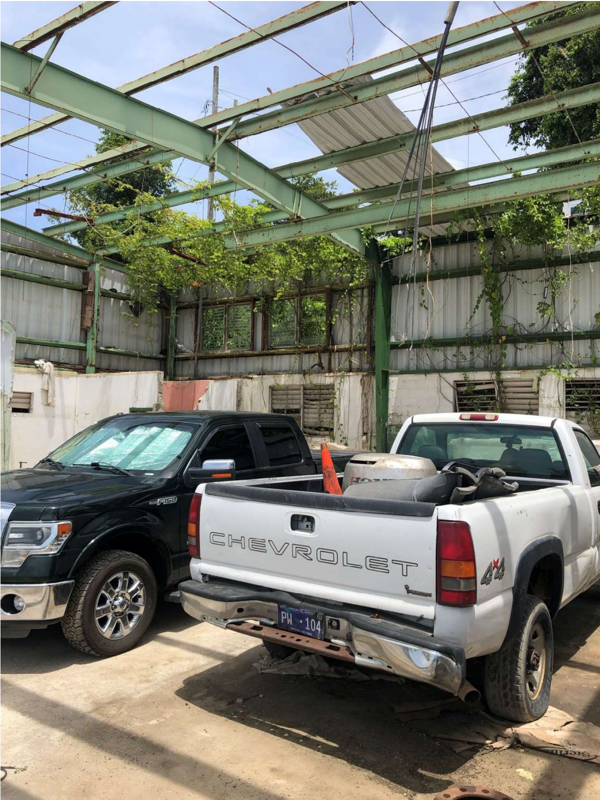
Figure 6: Hurricane Damaged Maintenance Building
