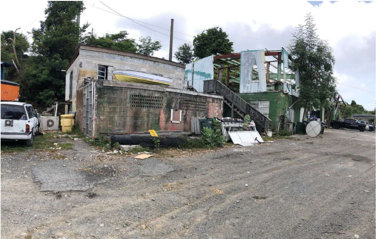
Figure 3: Hurricane Damaged Maintenance Building
