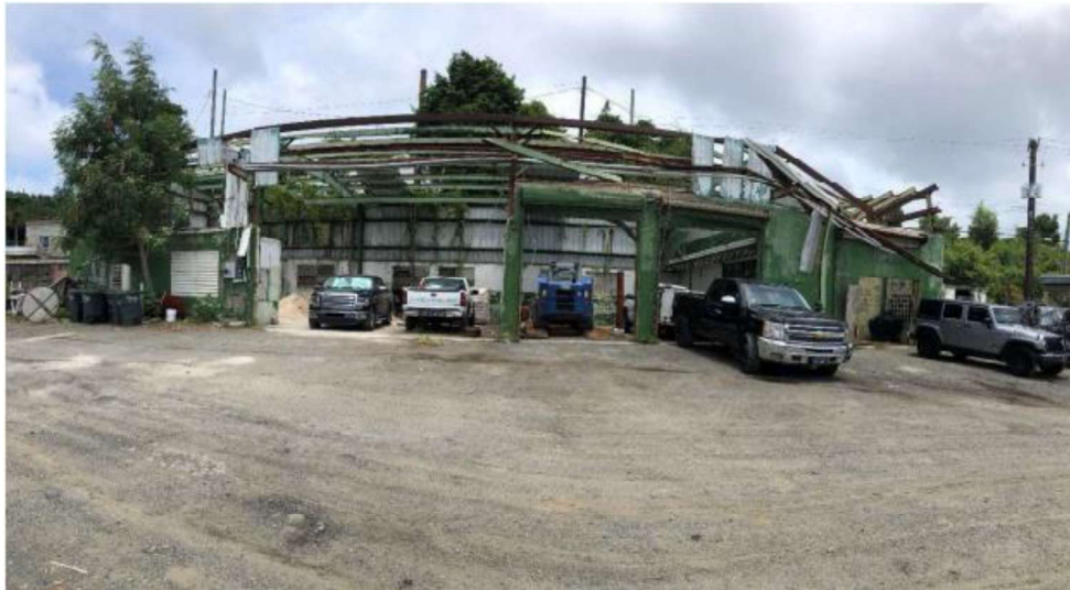
Photo of current site condition- hurricane damaged maintenance building
